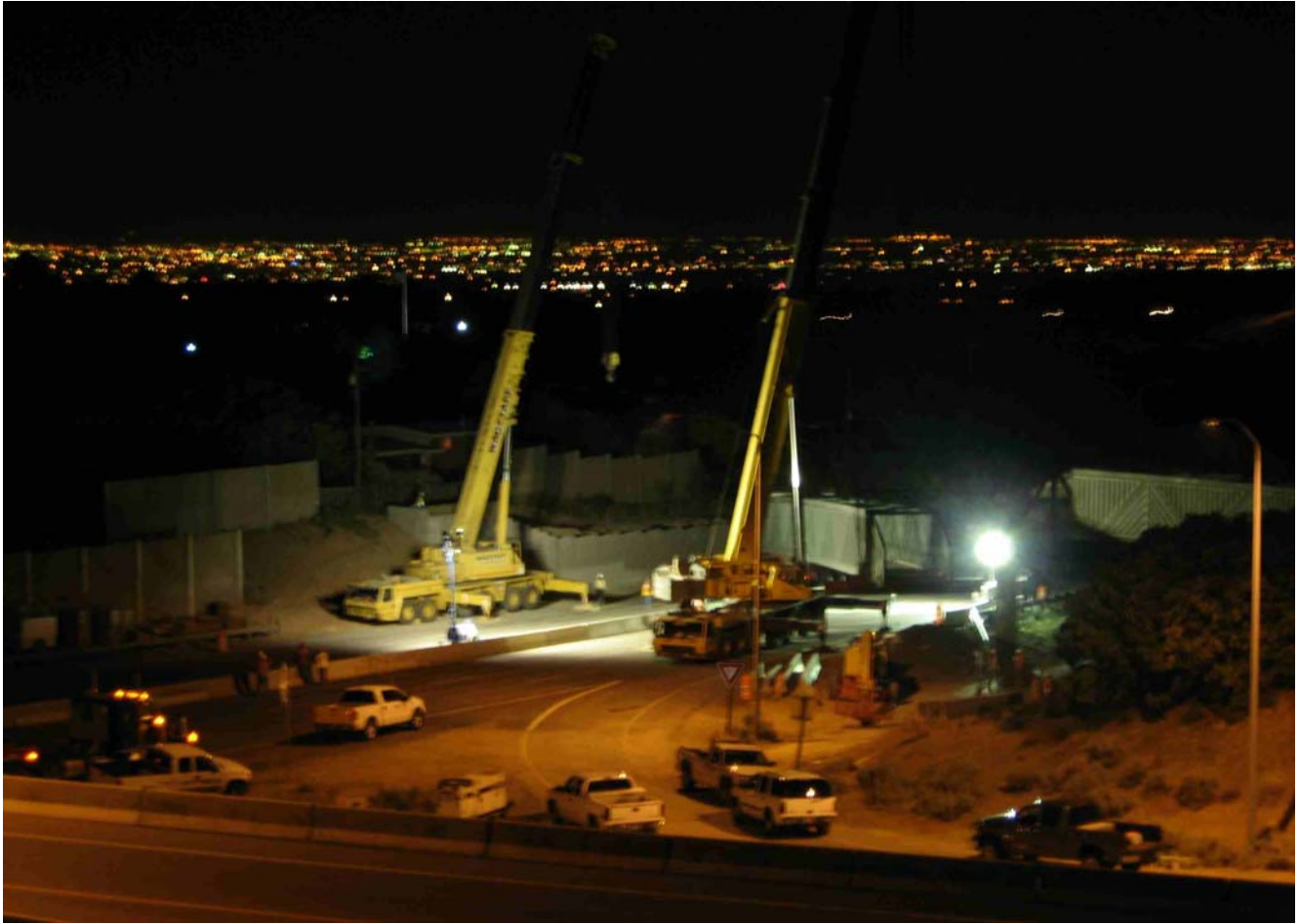
Bridge Placement Photos by Brian Roberts on July 8, 2007, 3:30 a.m. Pictures were taken from the small upper parking lot next to the trail-head.
